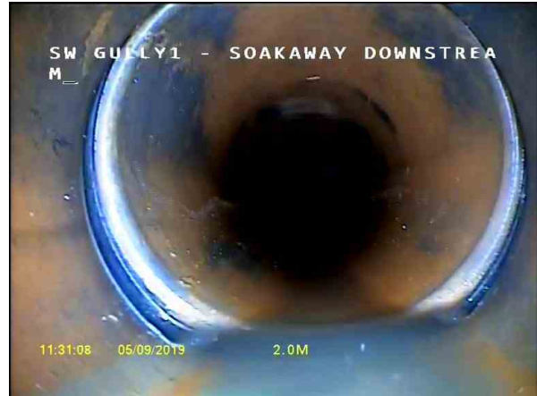
SW GULLY 1X_14c15926-64c0-4188-8db2-6eada36f77c6_20190916_151855_328.jpg, , 2.00m Joint displaced, large
