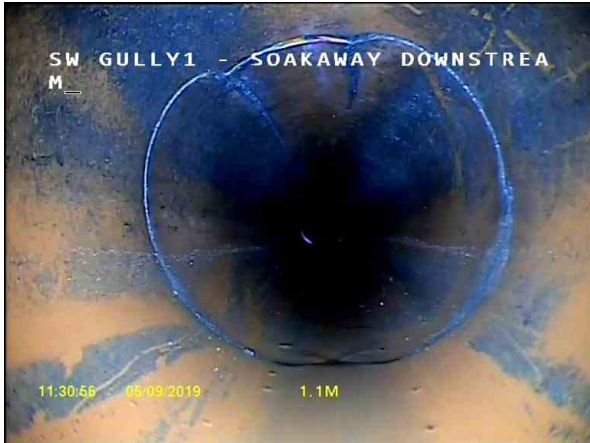
SW GULLY 1X_238bee7b-0ef1-40b3-94d9-e45fabb36af1_20190916_151849_054.jpg, , 1.10m Crack, circumferential from 12 o'clock to 12 o'clock
