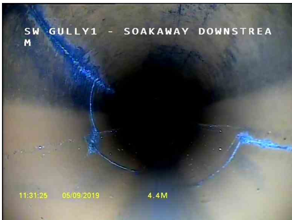
SW GULLY 1X_2ca956ba-7540-4b97-a6e8-a268fb3c04a2_20190916_151901_037.jpg, , 4.40m Cracks, multiple from 12 o'clock to 12 o'clock
