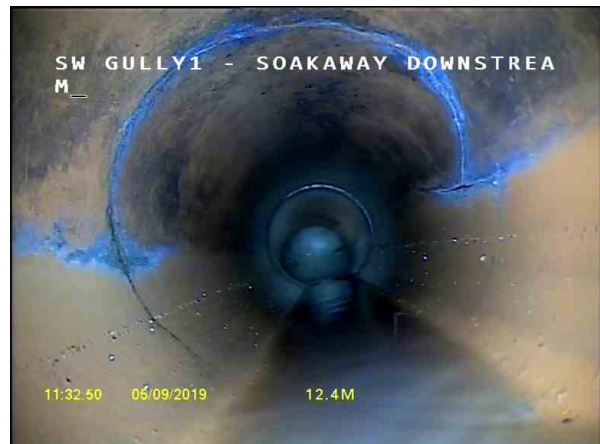
SW GULLY 1X_e573fd1b-45e8-46a8-8456-2c3663eb2edc_20190916_151921_263.jpg, , 12.40m Crack, circumferential from 12 o'clock to 12 o'clock
